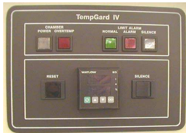
TempGard IV Panel
