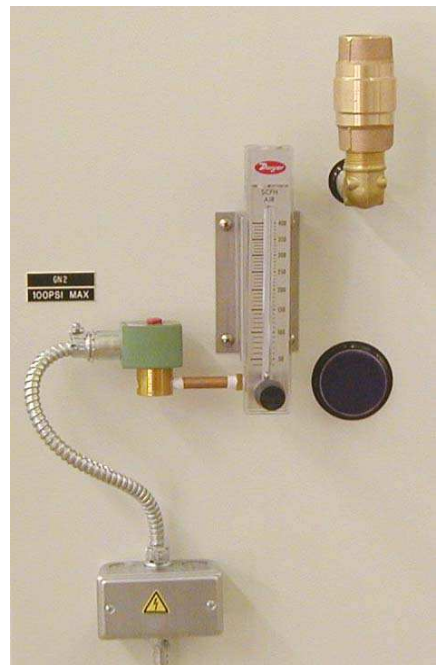
GN2 Purge System
