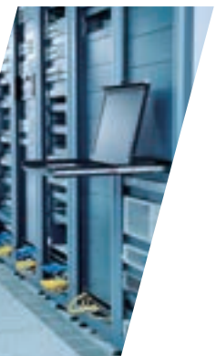
Control Room/ Data Center
