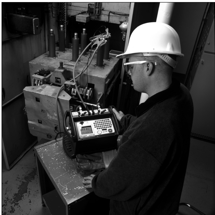
The DLRO600 shown measuring the contact resistance on a GE 15kV air breaker.
