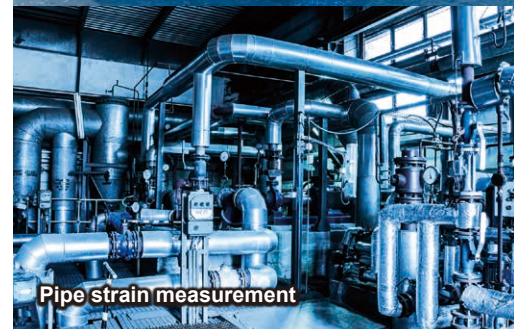
Brake and pipe strain measurement
