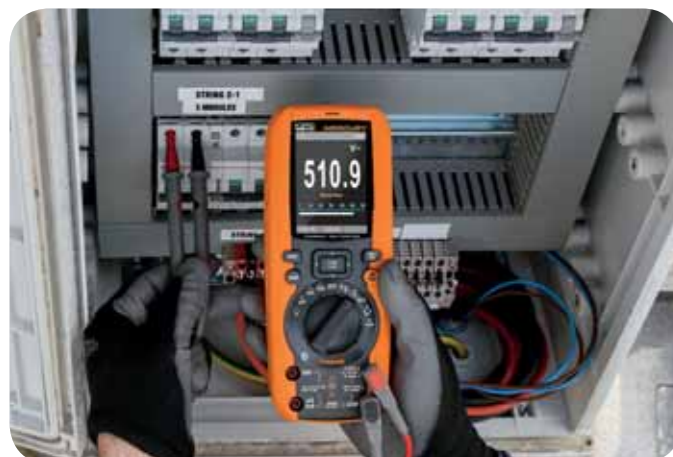
PV string Voc measurement
