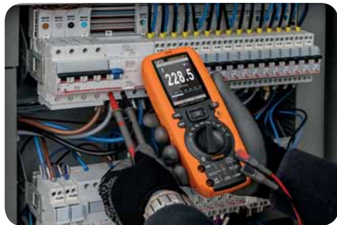
AC voltage measurement.
