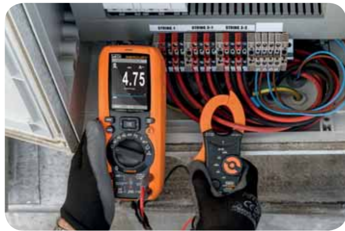
PV string Imp measurement.
