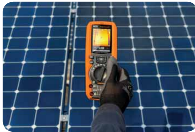
PV field thermography.
