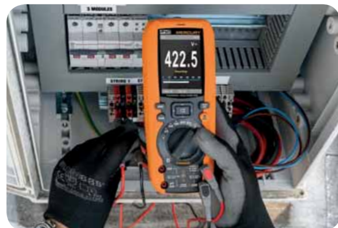
PV string Vmp measurement
