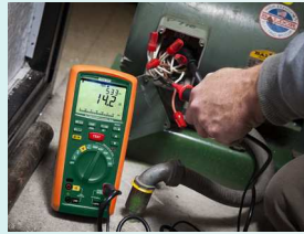
Insulation test on pump motor
