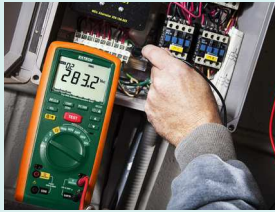
Voltage check on motor starter
