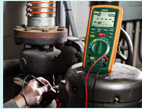
Insulation test on pump motor
