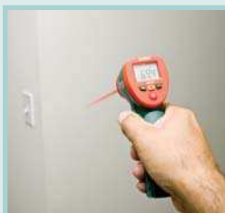
Check building for insufficient insulation
