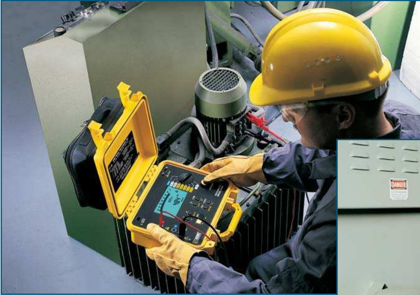
Model 1060 performing insulation test on contacts of a generator.
